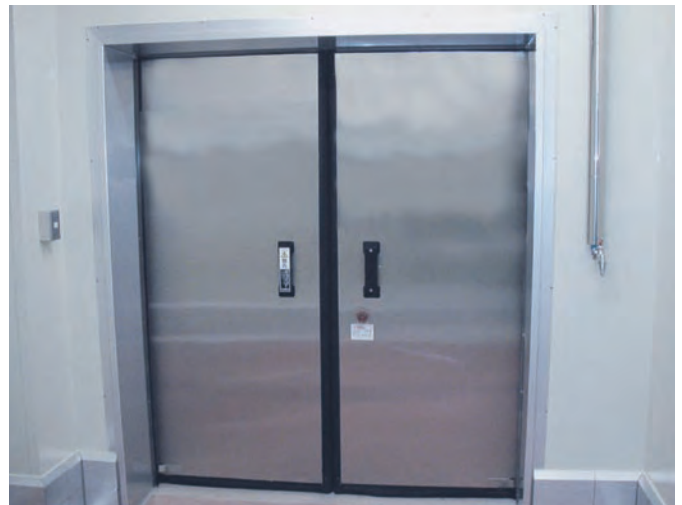
手動両引扉 (庫内) Manually operated double-leaf sliding door (interior)
